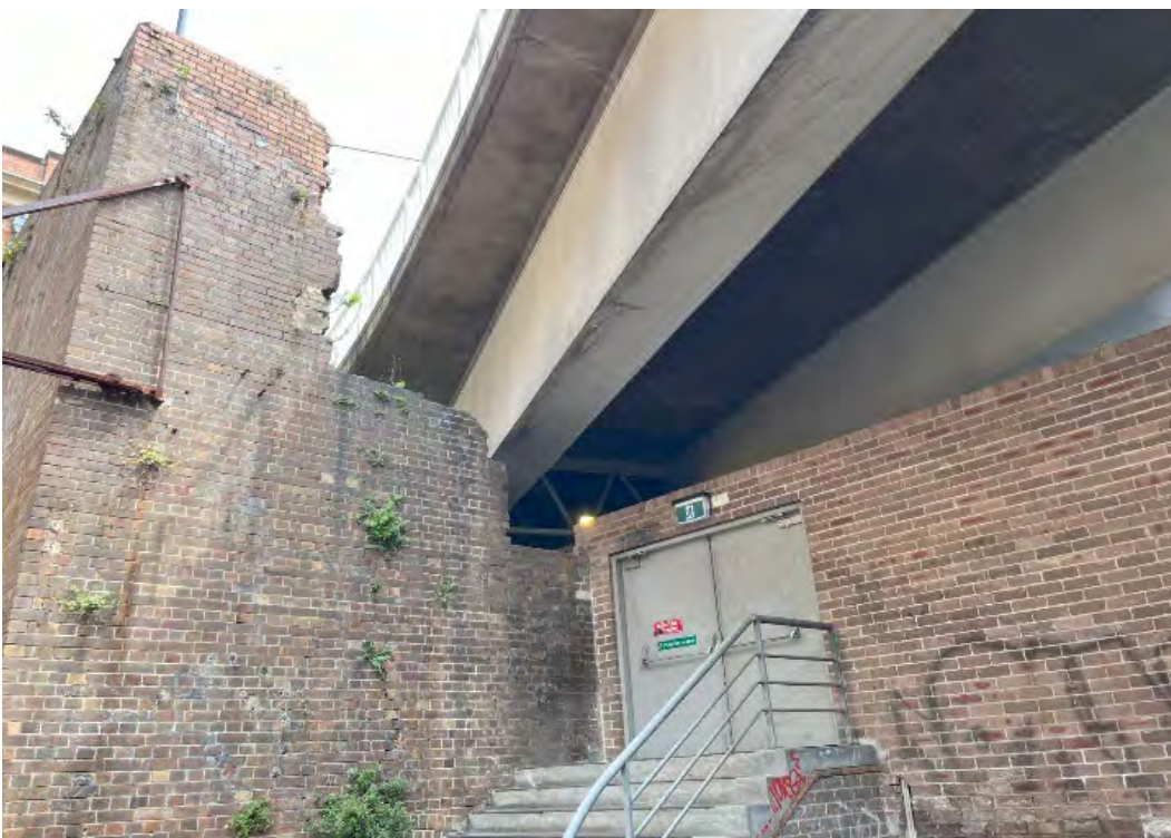
Figure 13 The remnants of the chimney stack (left) and the underside of William Henry Street (right)
