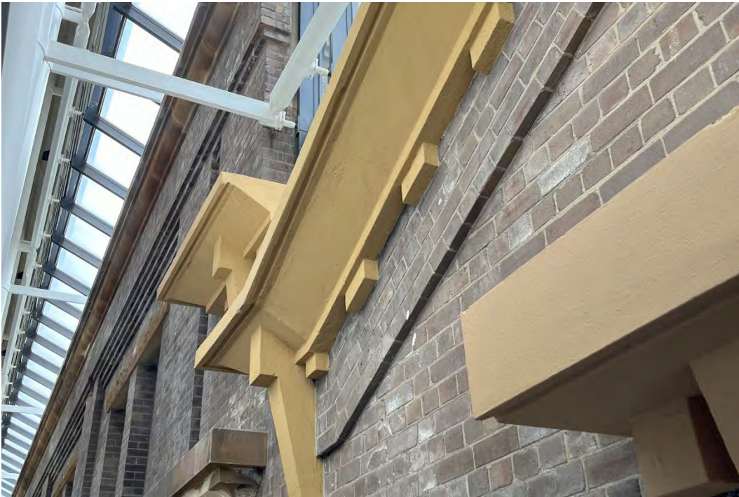
Figure 22 Detail of the interface between the Switch House and the Wran Building roof (Vault 1)
