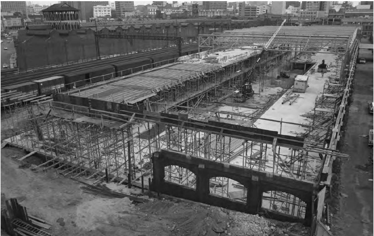
Figure 7 Works for the adaptive re-use of the Tram Depot underway, November 1980 Source: Powerhouse Museum Photo Library ST1D-SMN-16-12A
